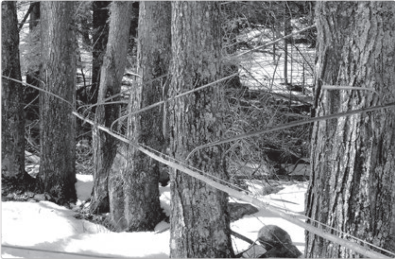
Figure 2: The Brower Sap Piping System, also known as the Gooseneck system, an early-20th-century all-metal tubing system. Photograph by Matthew M. Thomas.
